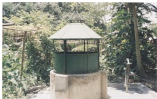
Fig. 5. Water-tank from which gravity feeds the houses
