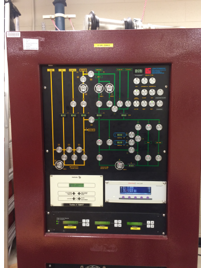
(b) Gas handling system panel
