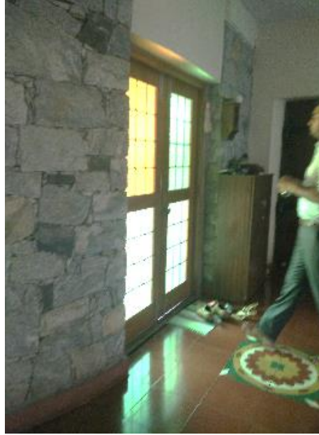
Figure 22. House 3 walls constructed with rubble masonry and no plaster.
