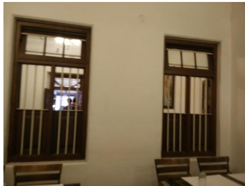
Figure 16. Internal windows present in traditional houses that help with movement of filtered air.
