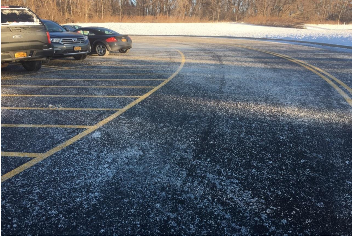
Figure 17. Observation of rock salt over applied in a commercial parking lot.
