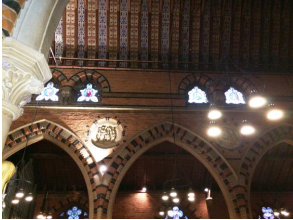
Figure 3.17 Misaligned clerestory windows and nave arcade from the interior.
