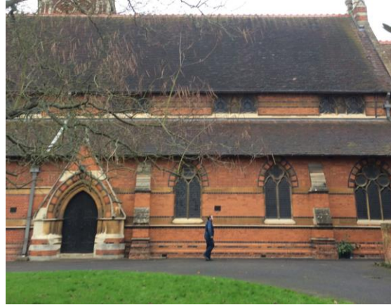
Figure 3.18 Misaligned clerestory windows and nave arcade from the exterior.
