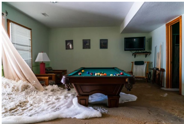
Figure 5.7. The effects of Hurricane Teddy within a rental beach house in Avon, North Carolina. (September 22, 2020)
