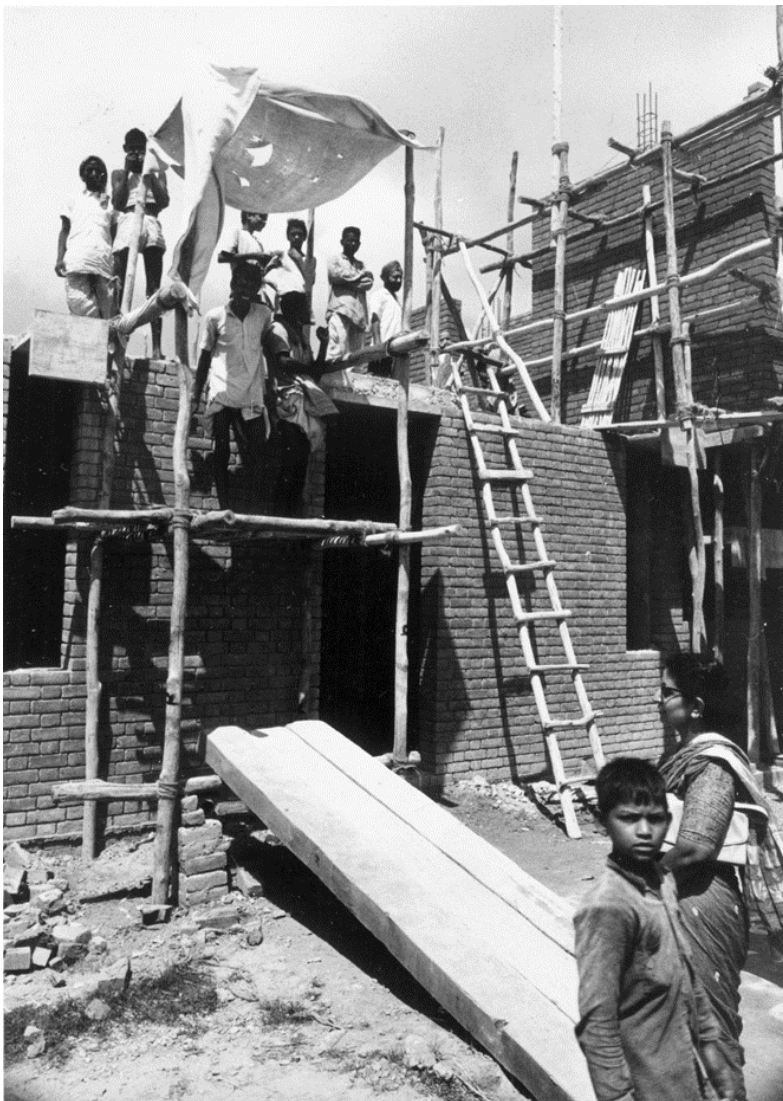
Figure 44: During the construction of Kanvinde residence, Akar, the construction was on a contract basis, as a result, Kanvinde's wife would oversee site work; [from the Kanvinde, Rai & Chowdhury archive]
