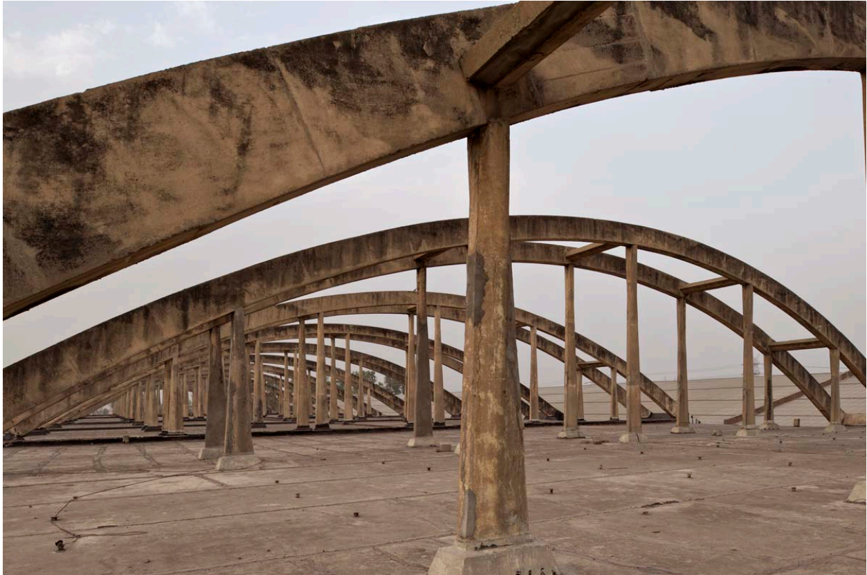
Figure 51: The structural system at Hindon River Mills; partnership of Mahendra Raj with Chowdhury; Photograph by Ariel Huber
