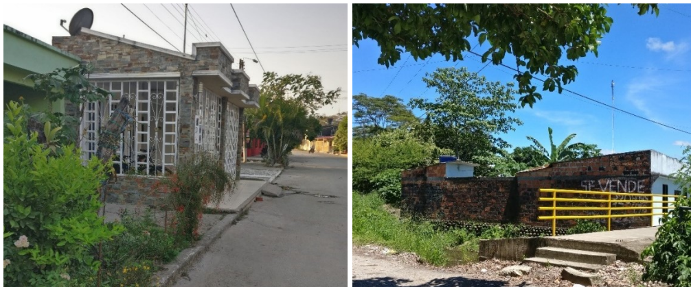
Image 3: Housing units in conflict with building regulations in neighborhoods El Popular (left) and Villa Union (right)
