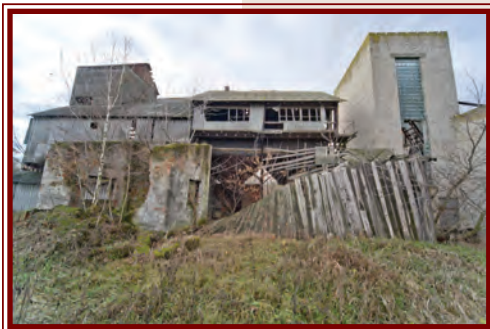
An abandoned building in the Chernobyl-restricted zone. (Source: Semion Shevtsov)
