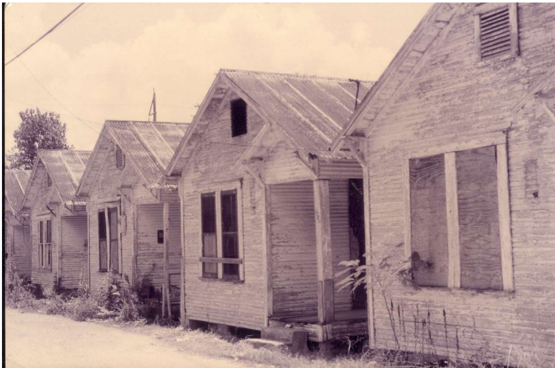
Figure 13 The original Row Houses prior to restoration. Photo by Sheryl Tucker Vasquez courtesy of Project Row Houses
