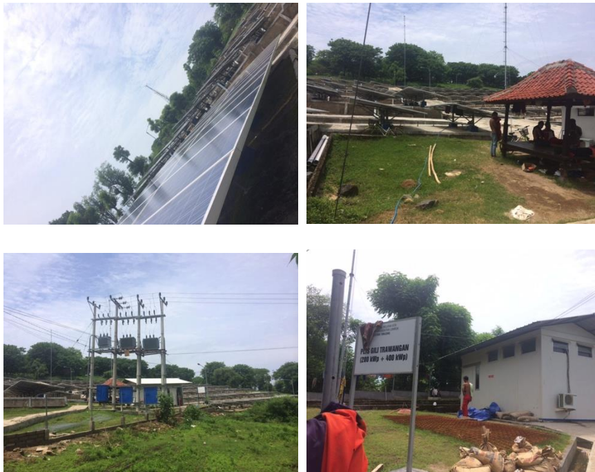
Figure 8. Photos of the 600 kWp solar power plant on Giri Trawangan, Lombok.
