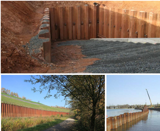
Fig. 2. Typical applications of sheet piling structures. In urban construction, they form retaining walls allowing for pre-foundation excavation (top) [14]. They provide slope stabilization in steep or uneven terrain (bottom left) [15]. In ecological applications, they are used for purposes like shoreline fortification (bottom right) [16].
