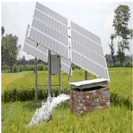
Solar Powered Irrigation Pumps
