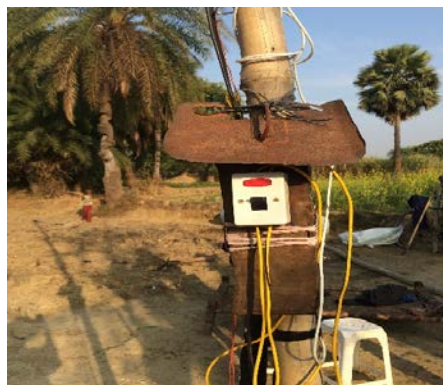
Electric Motor Pumps
