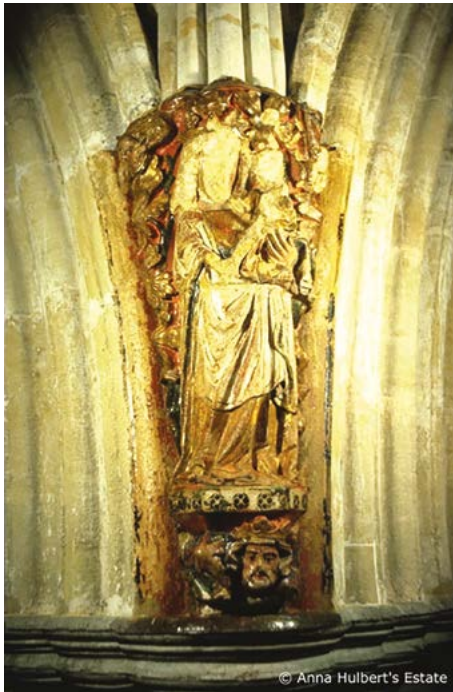
Fig. 1.29 Damaged corbel of Exeter Cathedral. Photograph by Anna Hulbert, no date. Image courtesy of Anna Hulbert's Estate. All rights reserved.
