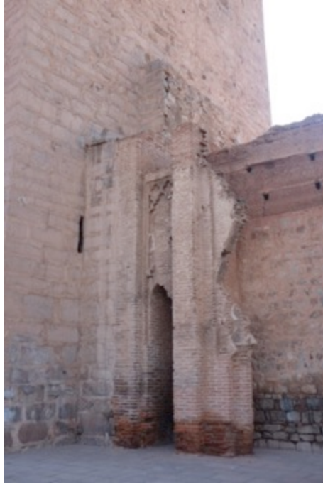
Fig. 2.19: Photograph showing the integration of the northern arcade with the base of the minaret. Photo author's own.
