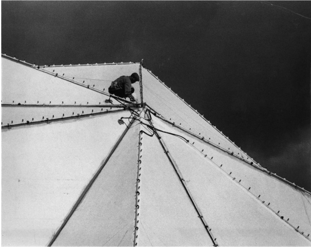
Figure 4.30. Installation of fog piping, Pepsi Pavilion, 1970. Reprinted from E.A.T., Pavilion (New York: E.P. Dutton, 1972).
