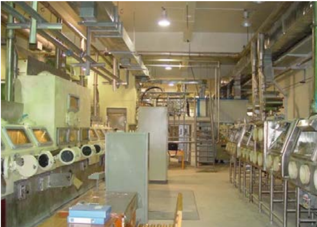
Figure 2.6: The Pilot MOX Fuel Fabrication Facility (0.5 tons/year) at Plant 404
