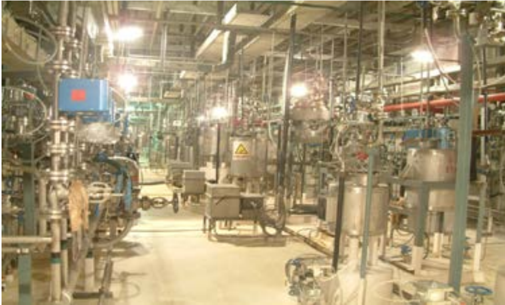
Figure 2.5: Inside of the Pilot Plant
