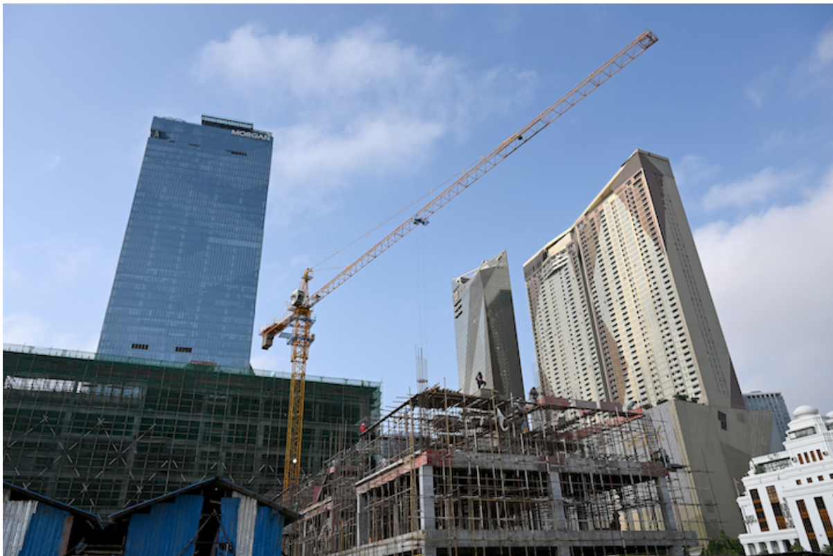
Building under construction in Phnom Penh on 17 March 2026. (Photo by TANG CHHIN Sothy / AFP)
