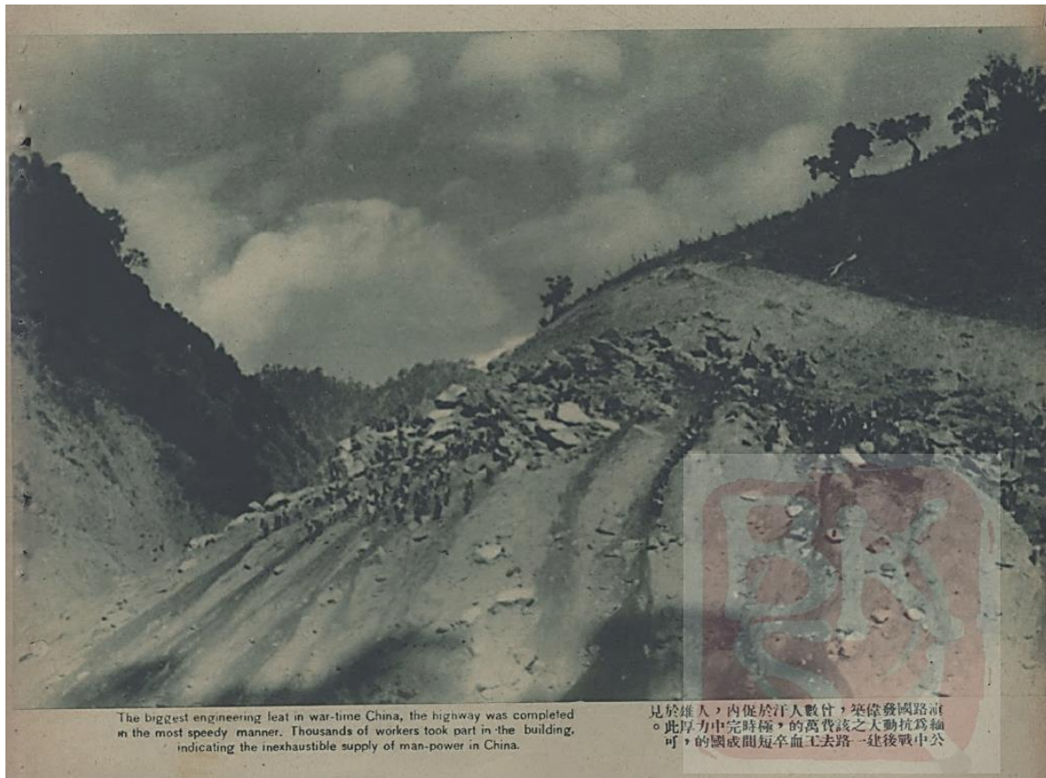
Fig. 16 Road builders seen on a steep slope. “From Kunming to Rangoon” 從昆明到仰光. The Young Companion 良友, Issue 154, May, 1940, n.p.
